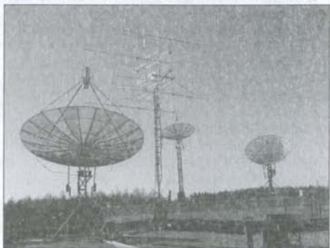
RW1AW's antenna farm
